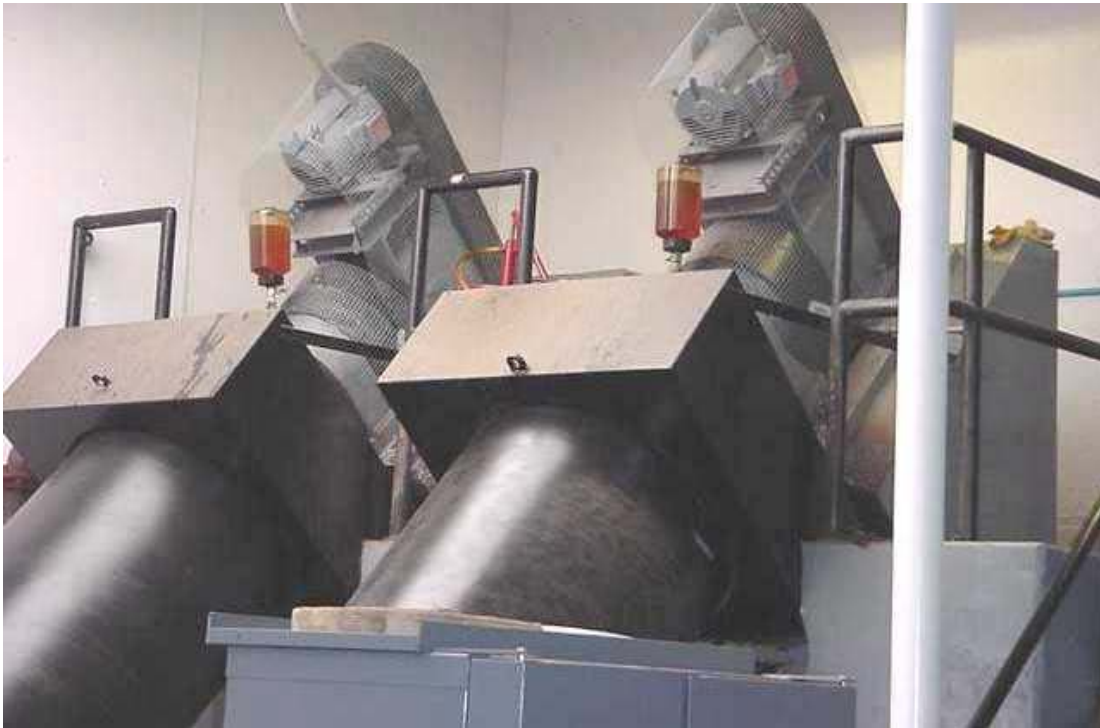
PHOTO 5-9 RAS Pump Motors
