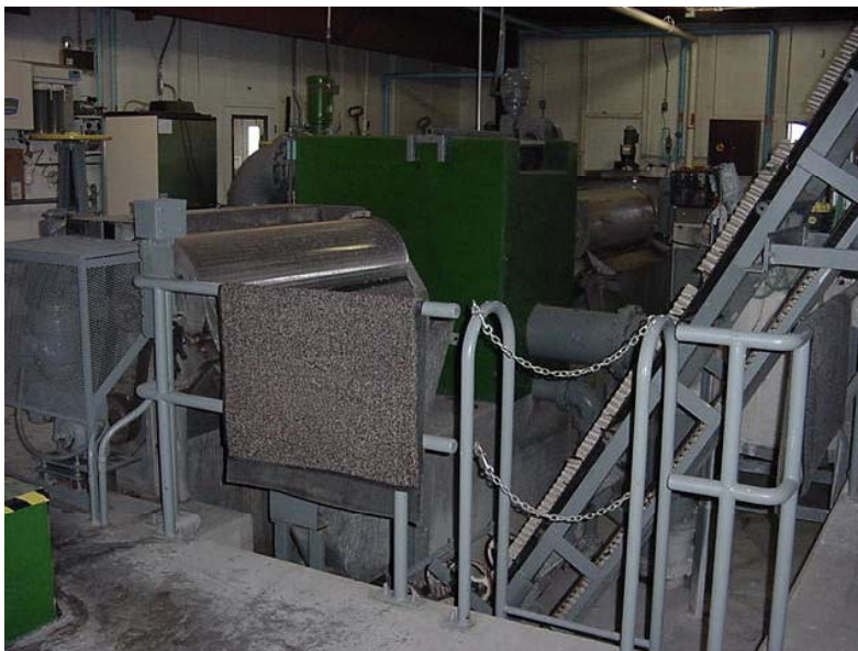
Influent Screening Area
