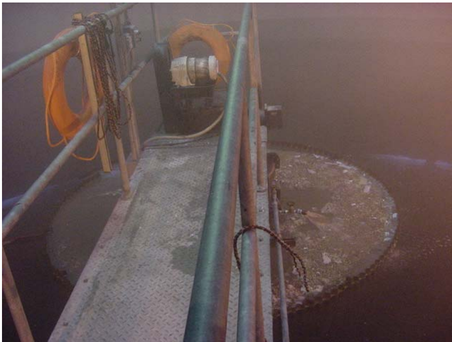
Rags and Scum Buildup in the Secondary Clarifier Centerwell due to Lack of Screening and Grinder Not Working Adequately
