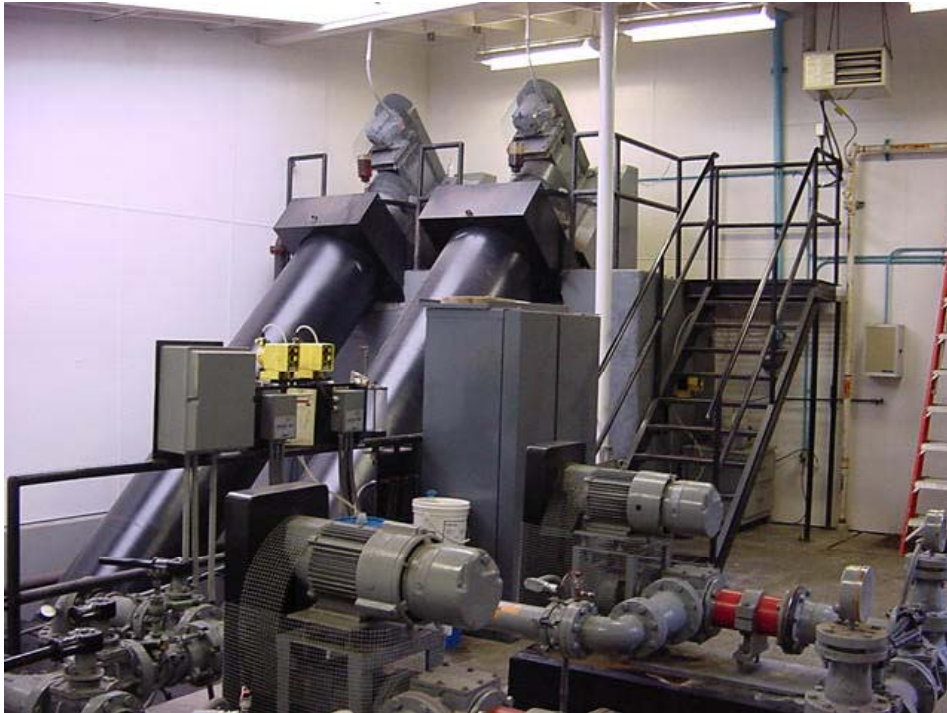
RAS Screw Pumps
