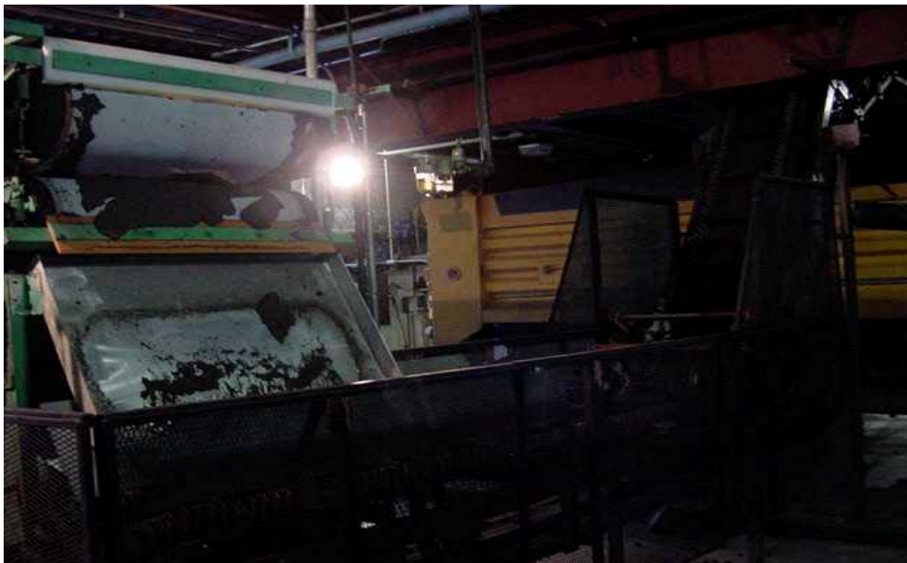
PHOTO 5-13 City of Kenai WWTF Belt Filter Press Dewatered Solids
