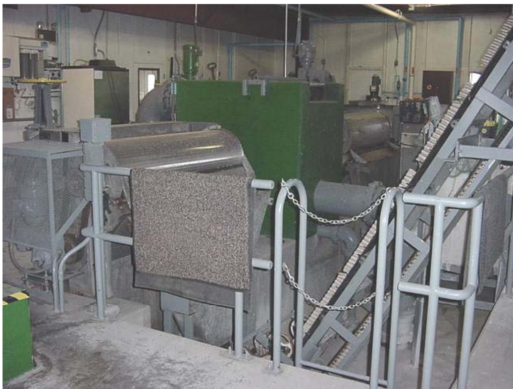
PHOTO 5-3 City of Kenai WWTF Existing Screens and Conveyor
