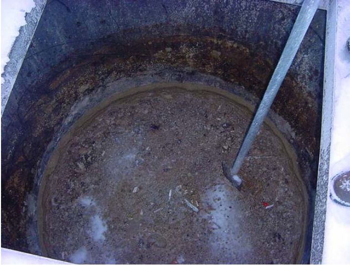
Grease Buildup in Influent Manhole
