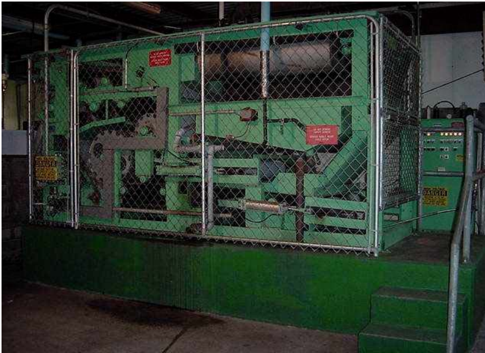
PHOTO 5-12 City of Kenai WWTF Belt Filter Press
