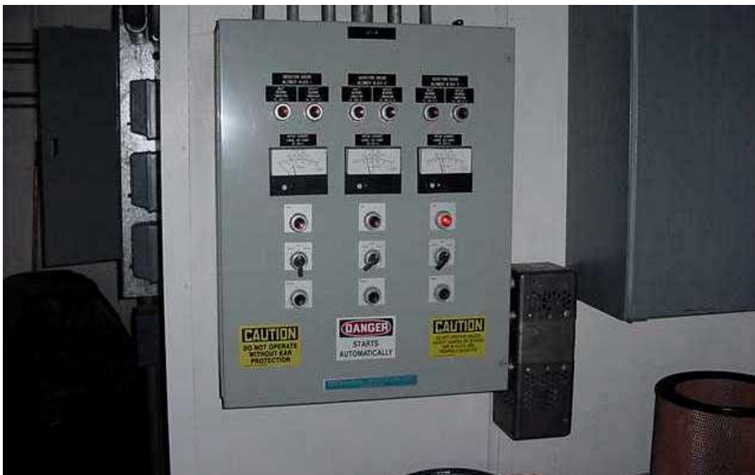
PHOTO 5-7 Aeration Basin Blower System Control Panel
