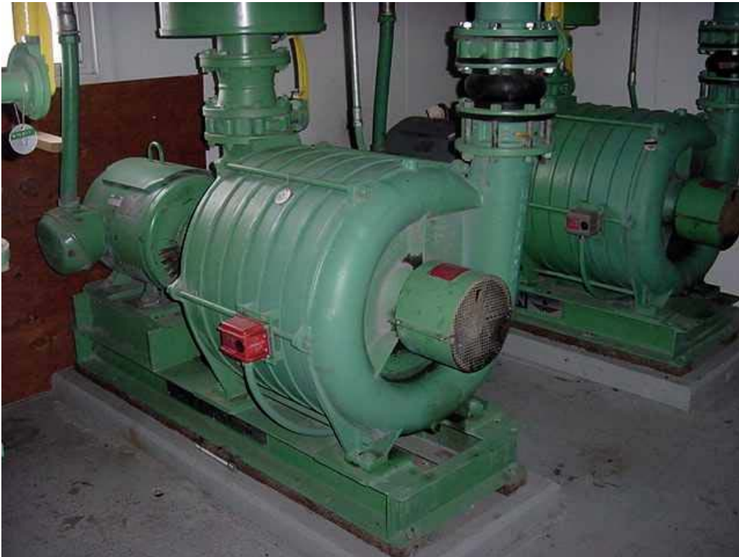
PHOTO 5-6 Aeration Basin Blowers
