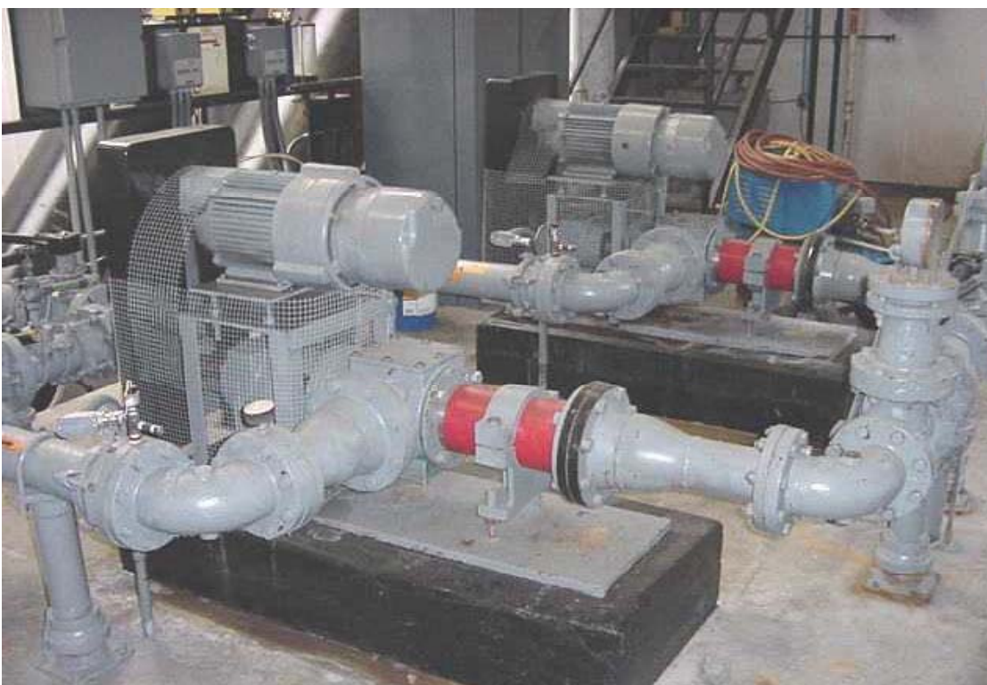
PHOTO 5-11 Existing WAS Pumps
