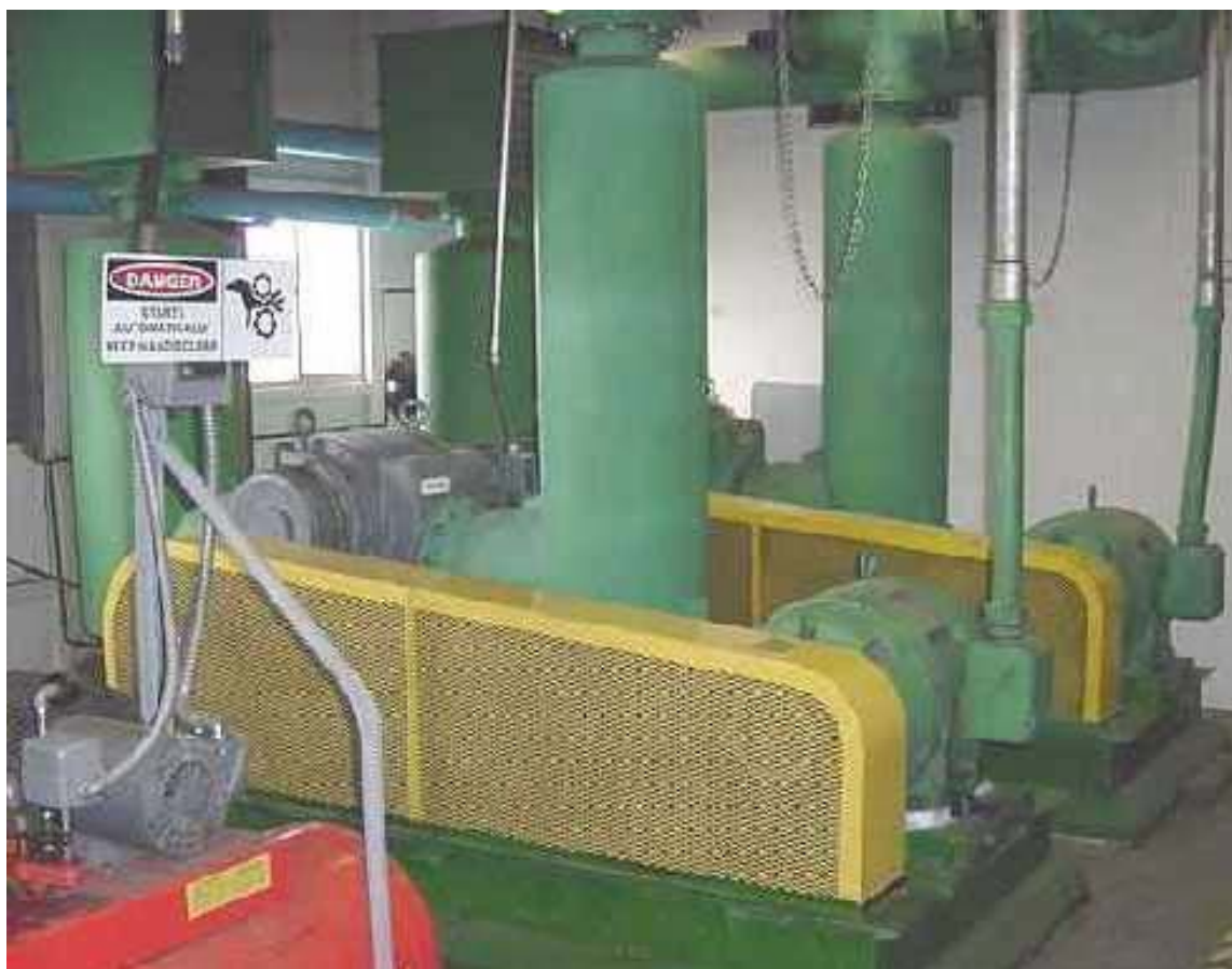
PHOTO 5-8 Existing Aerobic Digester Blowers
