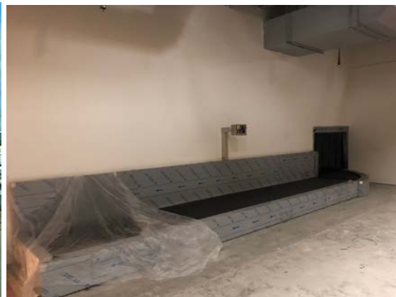
New Baggage Conveyor
