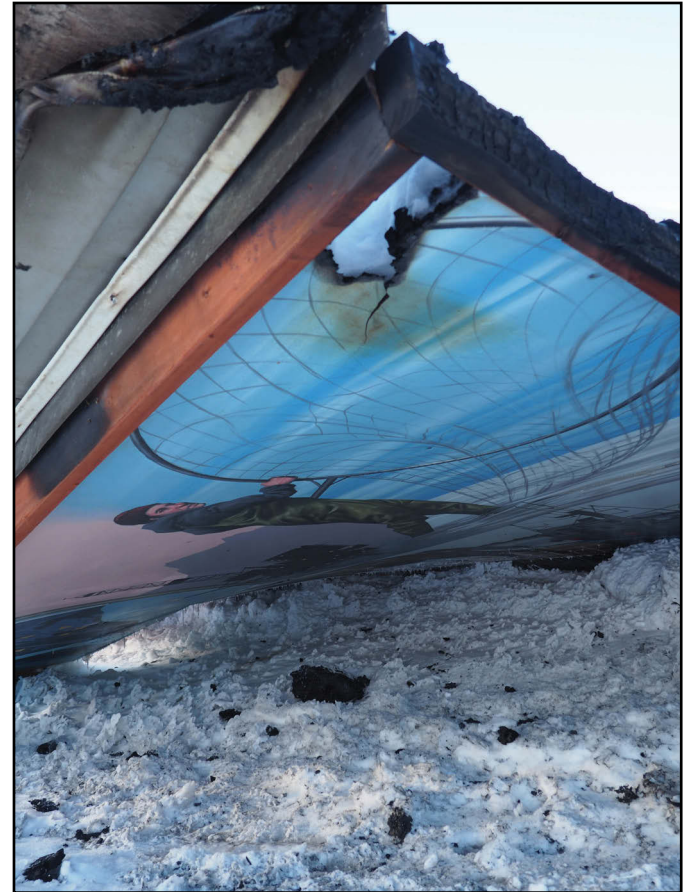
Exterior mural, following the fire, 2021.
