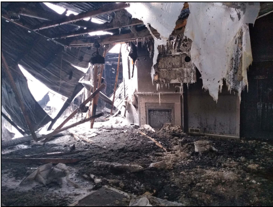
Triumvirate lobby after the fire, 2021.
